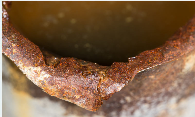
Hydrogen sulphide gas (H 2 S) is highly corrosive.
